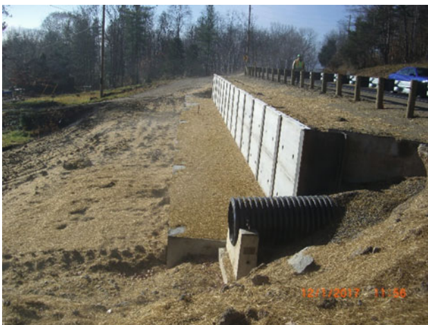
Fig. 10 Pile supported wall constructed along a highway in Ohio, to protect a road from an active landslide. A concrete cap connects two rows of steel piles, rigidly; on the right side of the cap, precast concrete panels placed between the piles' steel flanges to create a retaining wall
