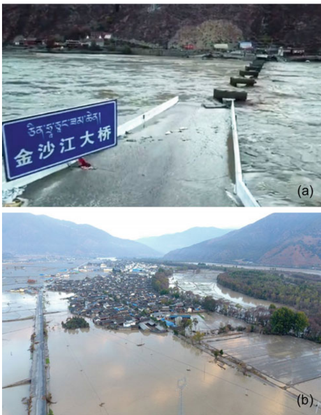
Fig. 14 Consequences caused by the dam-breaching flood: a damage to infrastructures; b flooding of densely populated communities (photo credit a Xinhua Net; b Dongfang IC)
