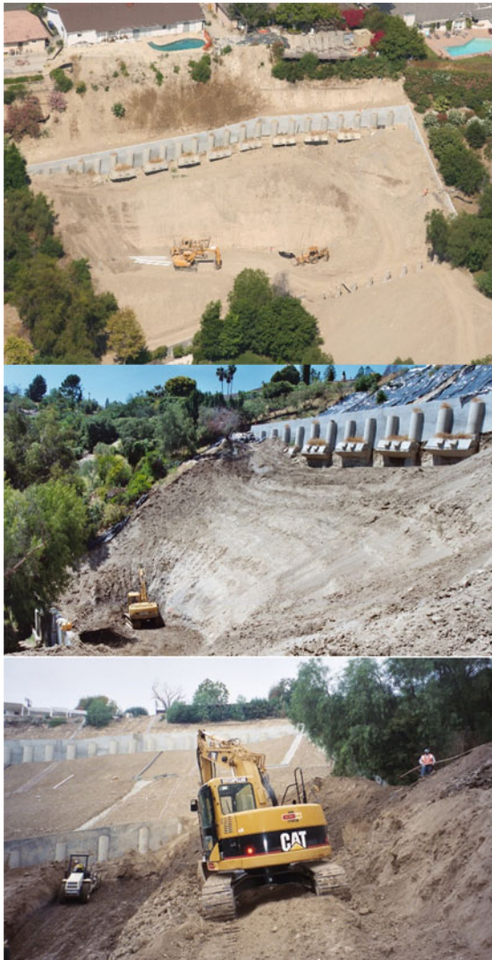
Fig. 2 Photos taken during a landslide stabilization in Encino, California. The project used two rows of stabilizing piles and tiebacks which allowed the completed removal and recompaction of the landslide
