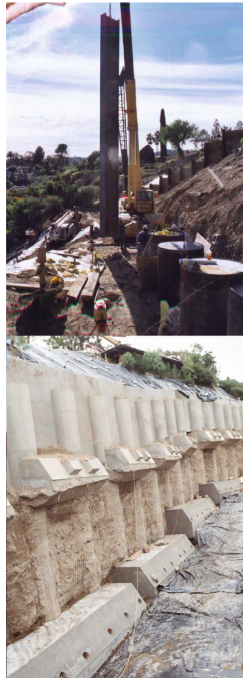
Fig. 3 Photos taken during construction of the drilled shafts and tiebacks shown in Fig. 2 (Top image: reinforcement of the drilled shafts with steel I-beams; Bottom image: exposed tieback anchor blocks during landslide removal)
