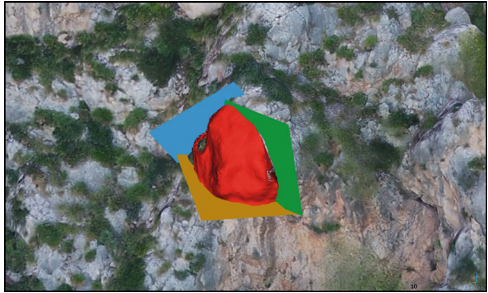
Fig. 4 Example of a potentially unstable block identified using the joint pattern characterized in the point cloud and extrapolated to cut the 3D mesh
