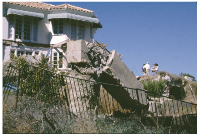
Fig. 1 Photo of a failed landslide stabilization in Calabasas, California. The project used a single row of stabilizing piles (drilled shafts) near the scarp that were insufficiently deep to resist the effects of the slide
