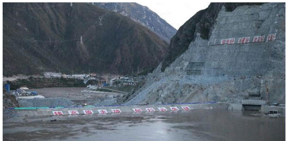
Fig. 8 The upstream cofferdam of the Suwalong asphalt corewall rockfill dam ( photo credit PowerChina)
