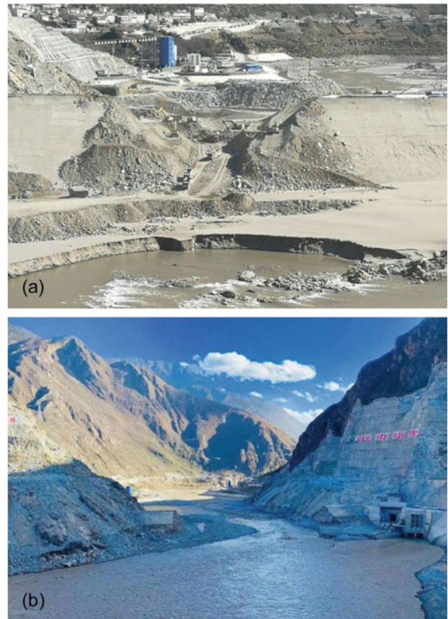
Fig. 12 Removal of the cofferdams at Suwalong to avoid hazard amplification: a removal of the upstream cofferdam; b after the dam-breaching flood (photo credit a, b PowerChina)
