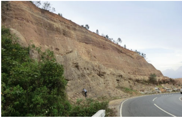
Fig. 1 Roadside residual soil overlaying with completely weathered rock (soil height is almost 18 m high)
