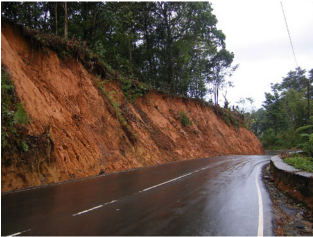
Fig. 1 Road cut slope, Saint Lucia primary road network, after landslide debris cleared (Photo: E A Holcombe)
