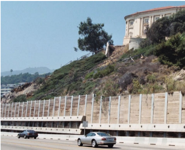
Fig. 4 Photo of a landslide mitigation in Malibu, California. Along the toe of the slope the project used piles and tiebacks to laterally support the landslide
