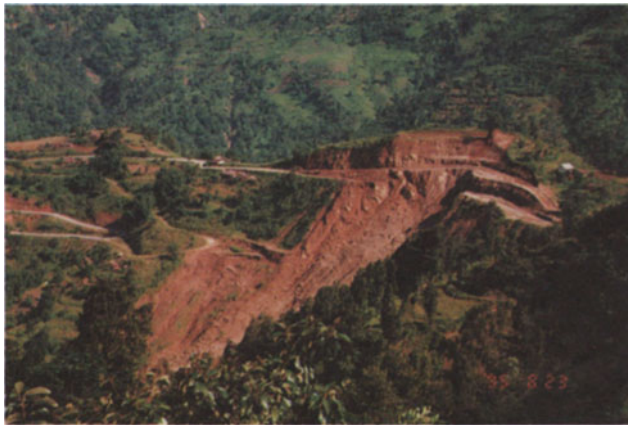
Fig. 7 Aerial view of the slope failure at station 62+000 km on the Charali-Ilam Road (Source Tiwari and Duarte 2013)
