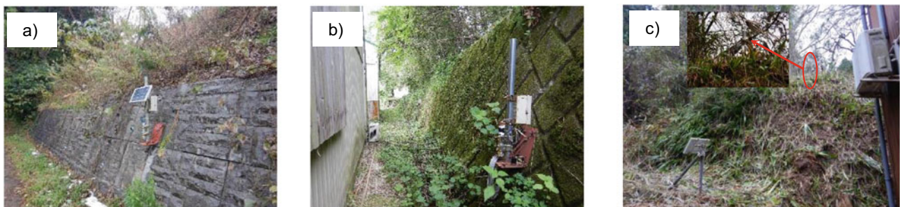
Fig. 6 Slope measurement/monitoring using POCKET, a block retaining walls along farm roads, b block retaining walls behind elementary school gymnasiums, and c slopes behind houses
