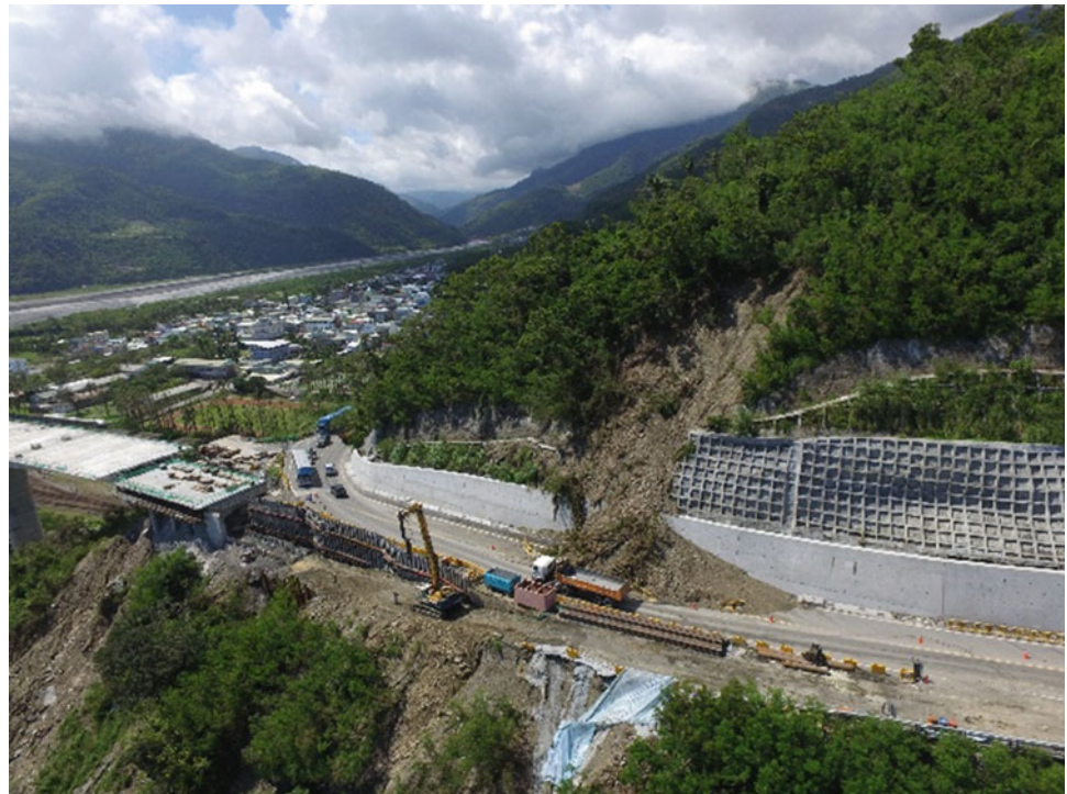
Fig. 9 Photo of route 9 413.5 k landslide
