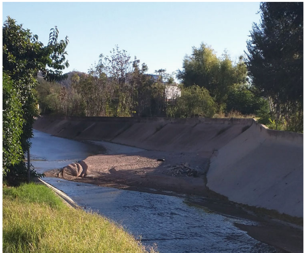
Fig. 8.11 Nogales Wash lies above the International Outfall Interceptor (IOI) (Photo T. Albrecht, with permission)
