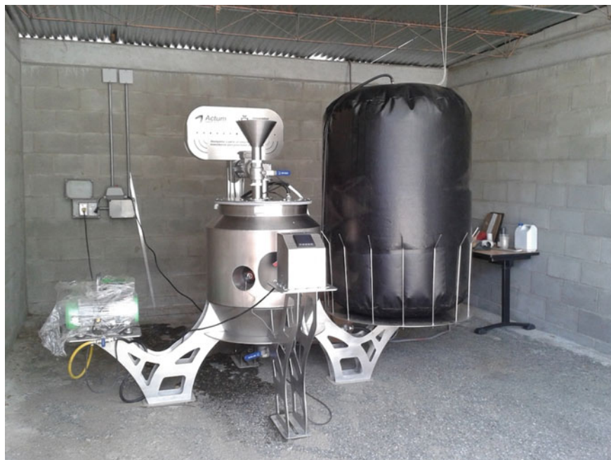
Fig. 3 Bio-digester UPB headquarters—Medellin. Picture provided by Oscar Vasco (2018)
