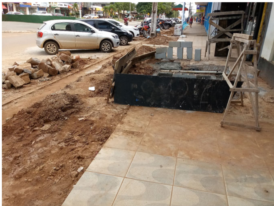
Fig. 9 Detail of a pavement in downtown Canaã dos Carajás, under repair. Source The author (2020)
