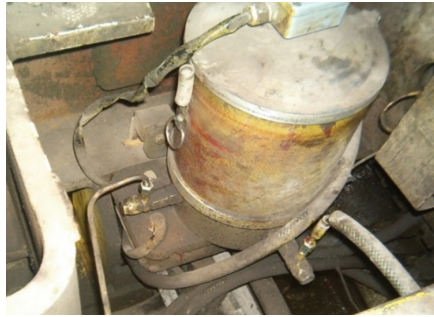
Fig. 6. Grease pump during operation.
