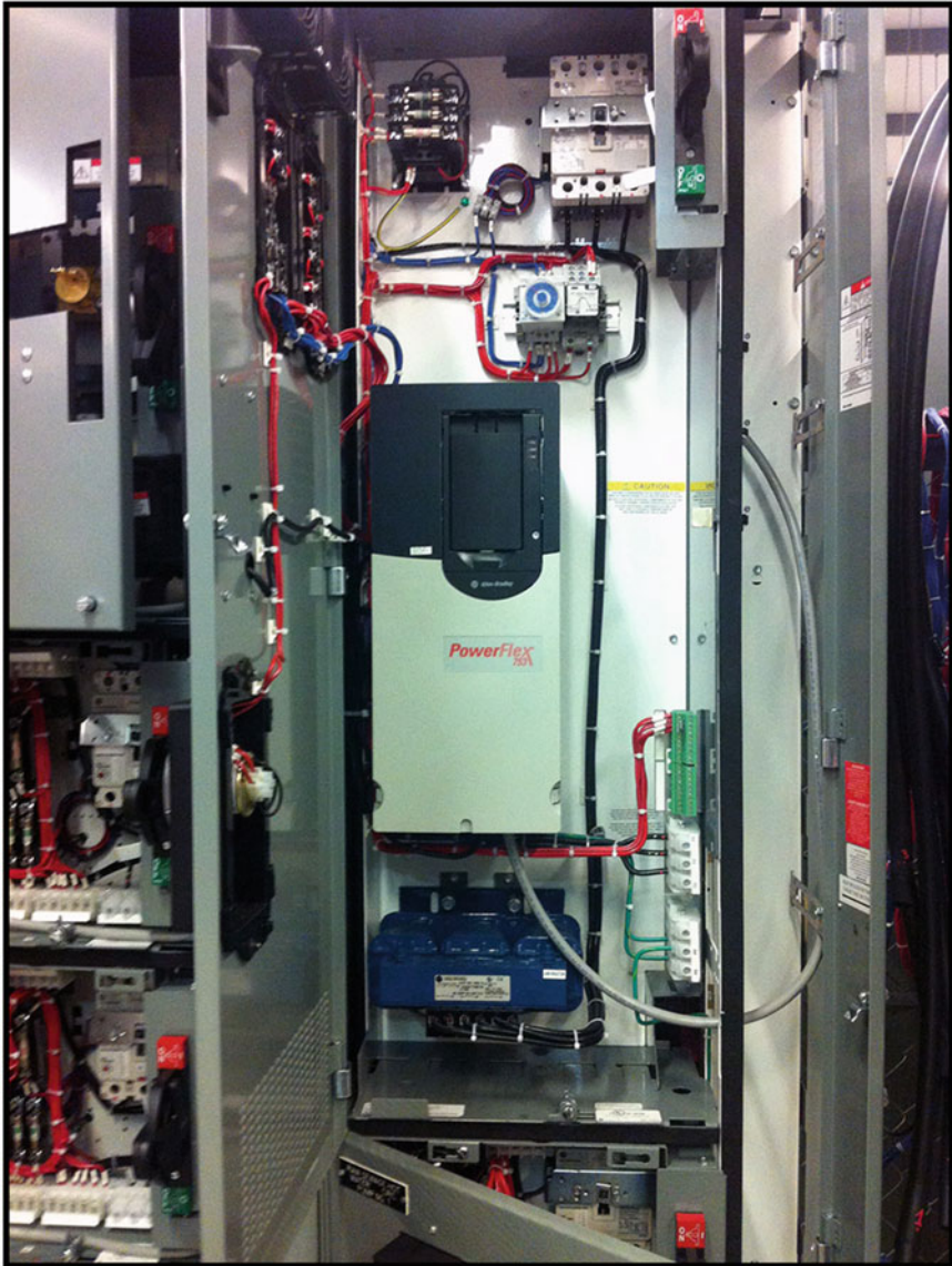
Fig. 1 Smart motor control centers (MCC) [13]
