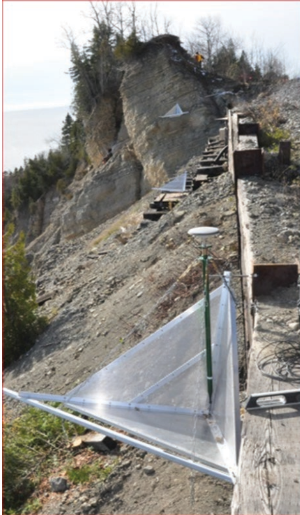
Fig. 1.2 Two metallic trihedrals installed on the retaining wall along the railway (1&2) and one on the tilted block (3). Reflector 1 shows a differential GPS instrument which provided measurements to validate the InSAR results
