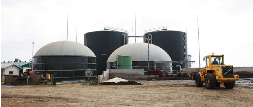
Fig. 2 Bio2Watt large-scale biodigester in South Africa (permission to use image provided by Thomas, 2019)
