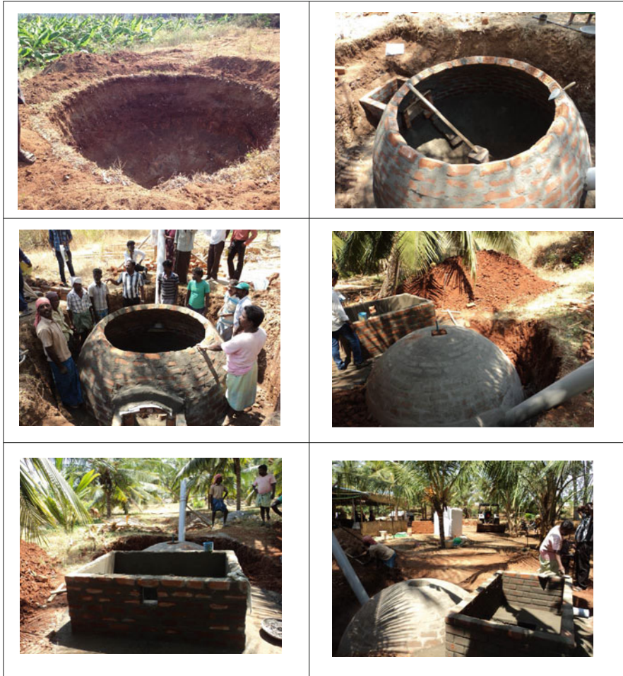
Fig. 5 The sequence of activities planned for construction of high solid-state biogas plant
