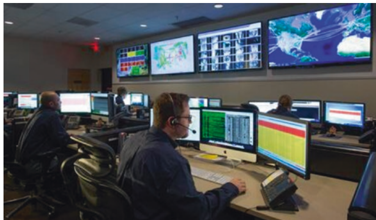
■ Fig. 15.3 Example of a Network Operations Center (NOC). (Image used by permission of NTT Ltd (available at ► https://www.gin.ntt.net/support-center/noc/ ))
