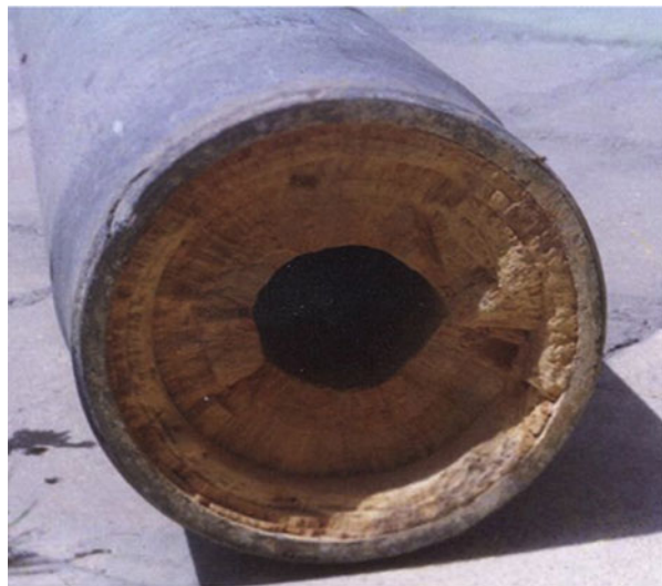
Fig. 2 Pipeline obstructed by scale of Ouargla city [2]
