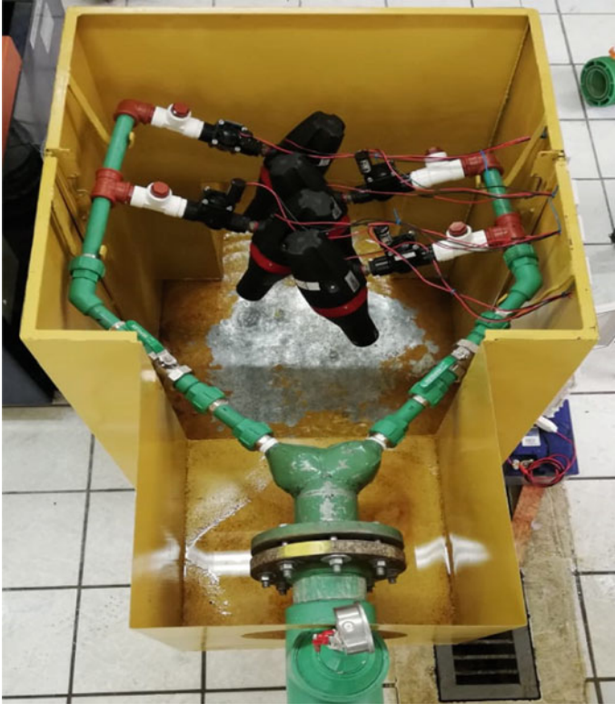
Fig. 6 Generation system installed in the pressure-breaking tank at UTPL Hydraulics Laboratory, top view
