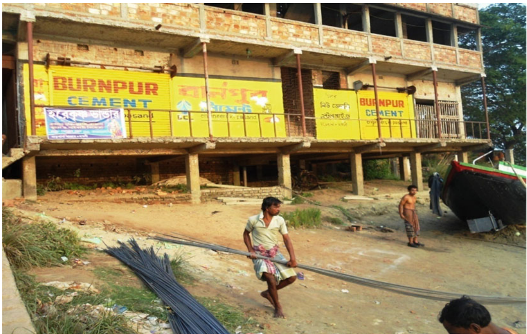
Plate 6.5 Encroachment of riverbed by the construction of commercial building at the confluence point of Darakeswar–Mundeswari in Marokhana, Hooghly
