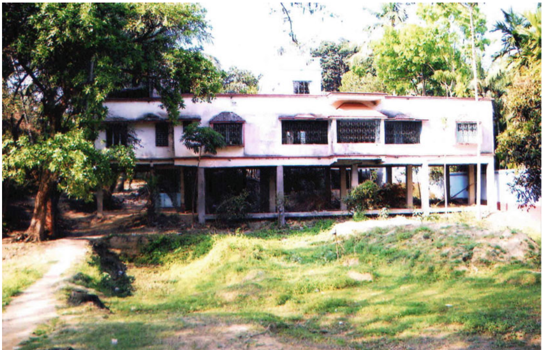
Plate 6.12 Structural modification of a school building (construction above 12 feet) for protecting the same from the ravages of flood in Khanakul-II Block
