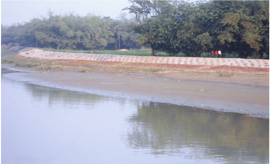
Plate 6.11 Partly concretization of the vulnerable left bank of River Mundeswari at the tri-junction point near Marokhana in Khanakul-II Block for preventing bank erosion due to tidal back-pressure of Rupnarayan River and high-velocity flow of Darakeswar
