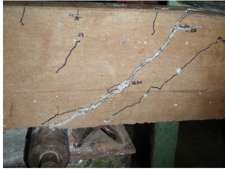
Fig. 5. The characteristic beams' destruction.
