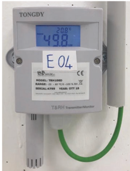
Fig. 2.8 (a) Cryo-room ventilation System Intake from top - Exhaust from Bottum (b) Temperature and Humidity sensor
