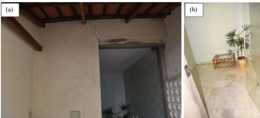
Fig. 16 Crack on the wall (a) and on the floor (b) of the entrance hall
