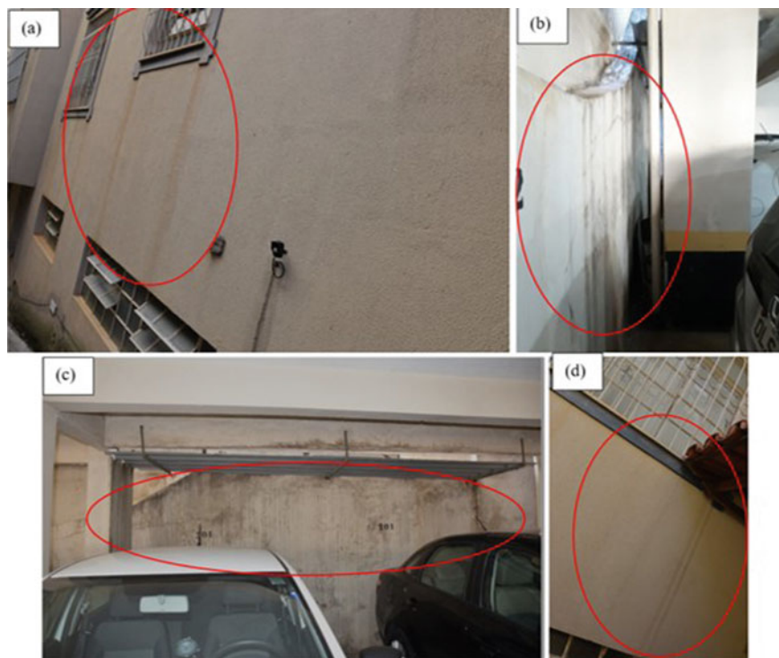
Fig. 18 Stains on the wall due to carrying dirt: a inefficient drips under the windows; b lack of drips above walls; c lack of waterproofing against the roof and stop of the garage and d lack of waterproofing of the encounter of the roof and wall of the building of the west facade of the building
