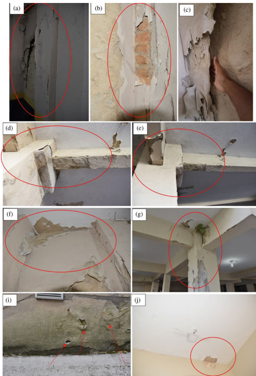
Fig. 20 Powdery disintegration of mortars and paintings: a–c on the garage walls; d–g encounter of slabs, columns and beams; h on the walls of the building close to the floor and i on the ceiling of the last floor (under the roof)
