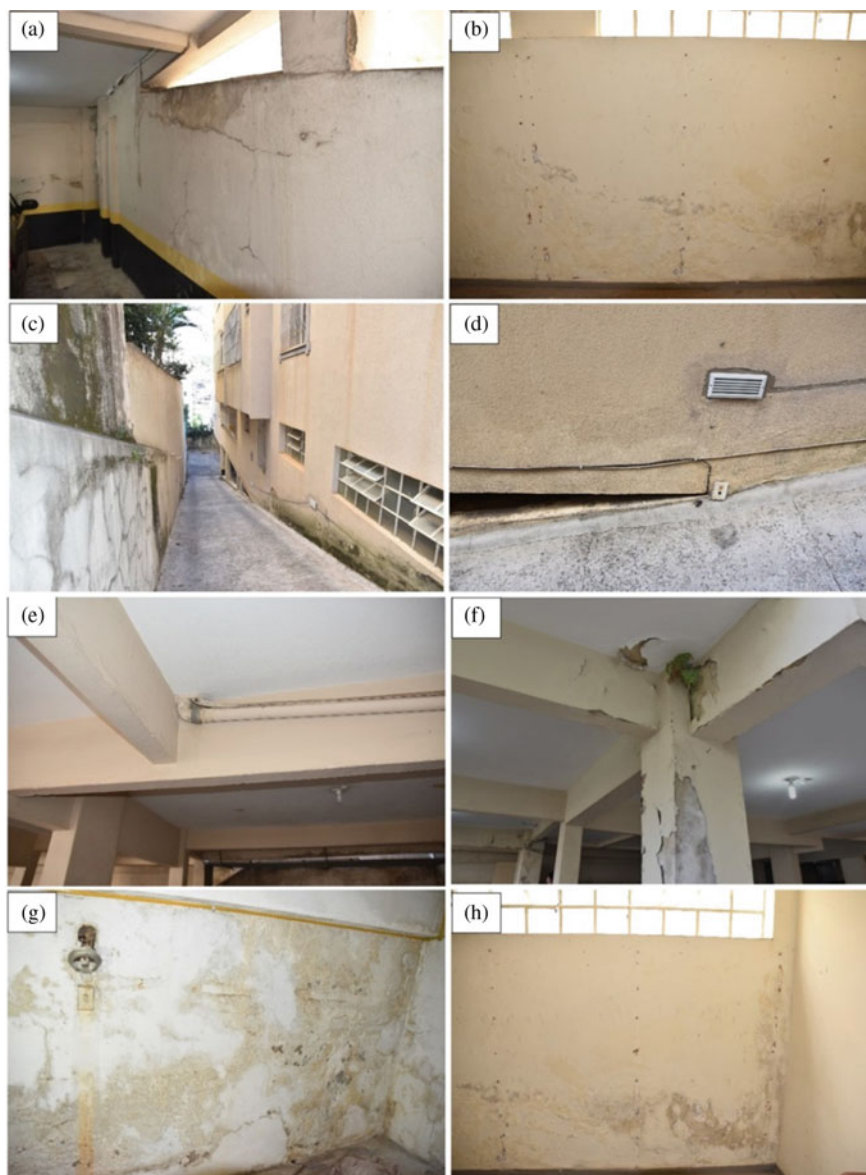
Fig. 12 Moisture from inefficient waterproofing on the access ramp to the garage and pedestrians entrance: a in the garage; b in the party room—garage ramp; c garage access ramp; d detail of the meeting of the ramp floor and building wall; e fixing and tightness of the pipe meeting to sewage drain in the encounter with the slab structure; f disaggregation and proliferation of vegetation due to the presence of moisture and use of contaminated aggregate; g basement in the 1st underground; h wall of the party room in the 1st underground
