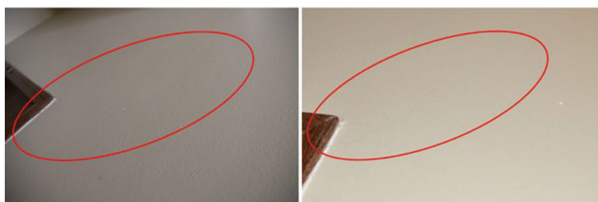
Fig. 25 Fissure at the corner of the door of top floor's apartment
