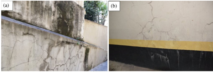
Fig. 19 Detachment of coating mortar and painting: a on the walls near the garage; and b on internal walls of the garage
