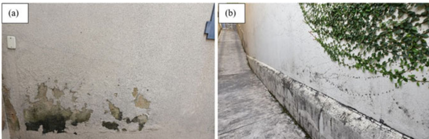
Fig. 11 Humidity from rain splashes: a pedestrian entrance; b garage ramp
