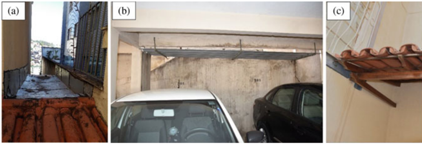
Fig. 10 Moisture from leaking roof: a and c pedestrian entrance hall; b garage
