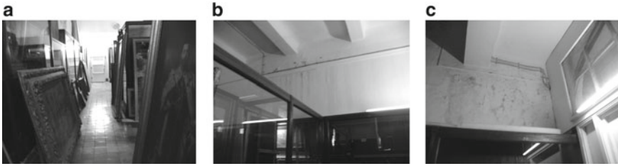
Fig. 3 a European painting store, b lime plaster wall and c wall dampness
