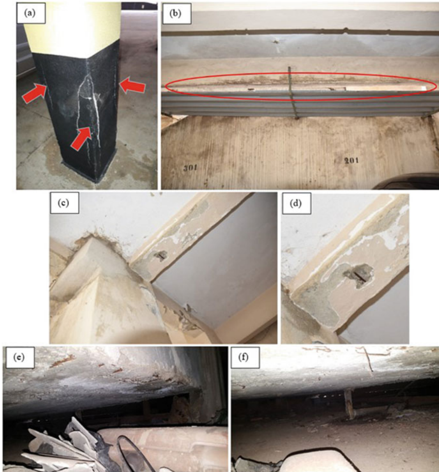
Fig. 14 Cracking and swelling of structural elements in the building’s garage: a column; b beam; c exposed reinforcement on the beam; d detailing of the exposed reinforcement and e and f detailing of exposed reinforcement of the upper reservoir
