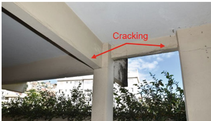
Fig. 13 Horizontal cracks in the columns at the back of the building's garage
