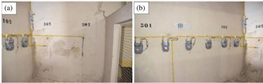
Fig. 30 Location of gas measurer: a side view; b front view
