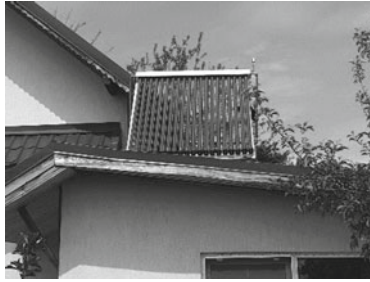
Fig. 3.7 Photo of a BAST on the roof of a house marking the lack of compatibility between the equipment and the building due to the wrong solar orientation of the house
