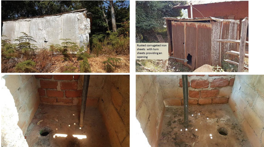
Fig. 2.10 Kikoo project toilet details: (a) Catholic primary school toilet, (b) community center toilet with torn wall and degraded external enclosure, (c), (d) internal view of the Catholic primary school toilet with intact walls, sunlight rays on the floor, squatting hole, and ventilation pipe installed on concrete floor
