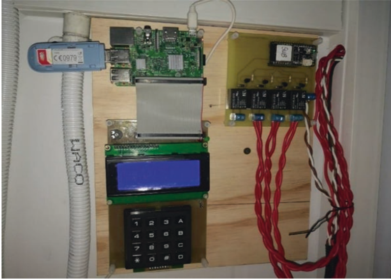
Fig. 3.23 Secured smart home switching system smart hub and smart switchboard implementation
