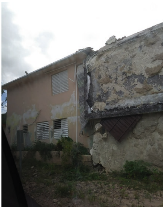
Fig. 10.13 Visual mold on the exterior of a post-hurricane residence in Utuado, Puerto Rico. (Permission granted by photographer Tyler Turner)
