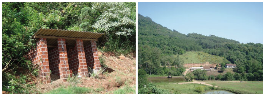
Fig. 4.5 Poorly constructed structures that compromise the environment close to the farms (a) unsecured compost for animal entrances and deteriorated and (b) poultry construction close to cisterns and rivers. (Authors, 2019)
