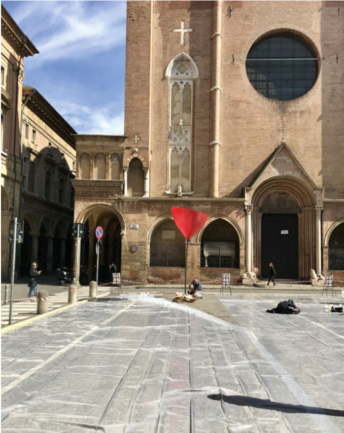
Fig. 5 Self-construction workshop reportage. Day one: safe delimitation of the area and coverage of the asphalt paving with a plastic sheet
