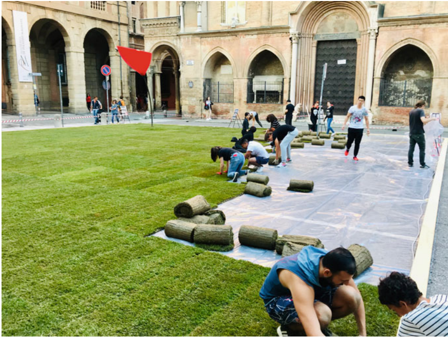
Fig. 6 Self-construction workshop reportage. Day two: installation of the flower light element and application of the rolls vegetable meadow
