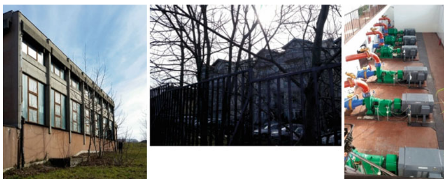
Fig. 1 Pumping station No. 25. “Mokroluško brdo” in Belgrade (left), residential building in the nearby the pumping station (middle), and distribution of the water pump engines in the technical room inside pumping station (right)
