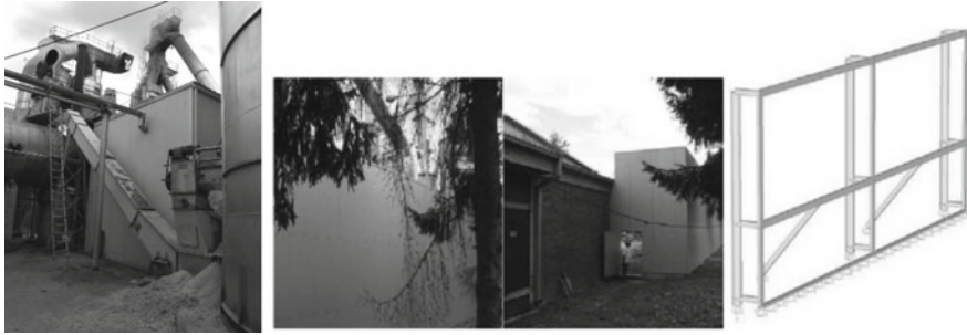
Fig. 4 Elements of the noise protection system in the “SPIK Ivanjica Fantoni Group” plywood factory
