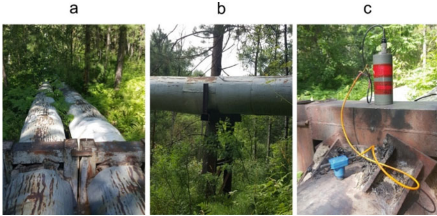
Fig. 1 a Pipeline section with rigid pipe fastening to the support b pipes laid on the rack without rigid fastening recorder and c geophone mounted on the pipe
