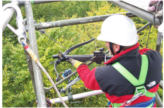
Fig. 6.9 Installation of a 45-m walk-up tower in a beech forest in Thuringia, Germany (photo © Martin Hertel, MPI-BGC)
