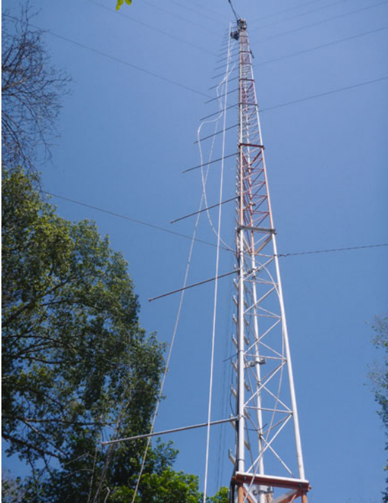
Fig. 6.10 A 36-m triangular mast near Tanguro, Brazil, during the installation of isolated lightning protection wire (photo © Martin Hertel, MPI-BGC)
