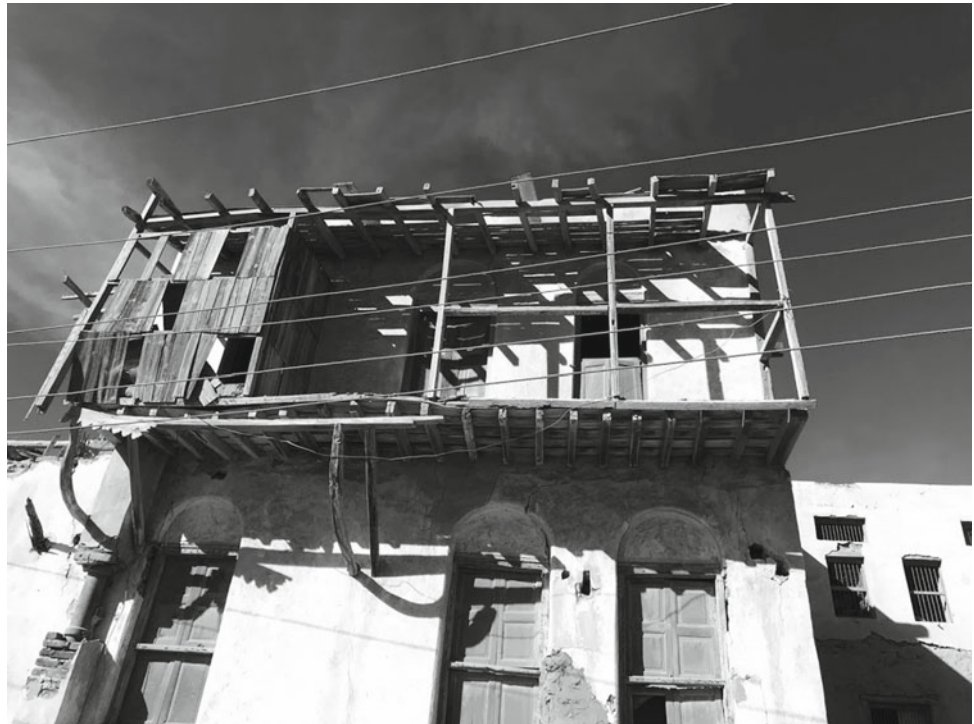
Fig. 25.8 Deteriorated old house more than 100 years old. Source A photo by Author
