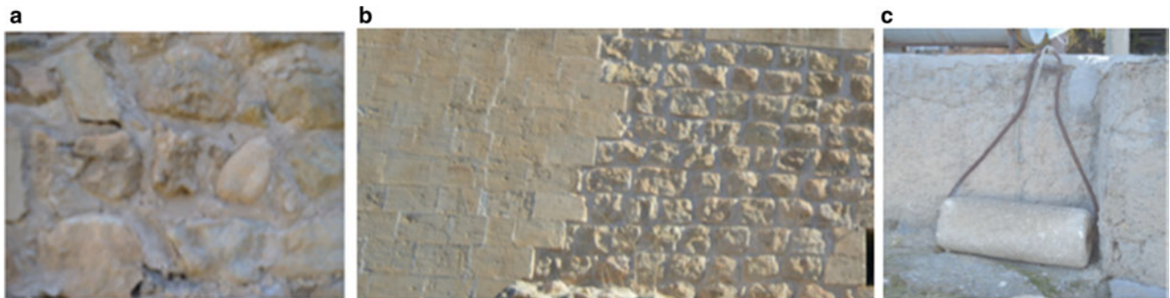
Fig. 13.9 a Cas mortar (left), b different techniques used on the same façade (middle), c gundor (right)
