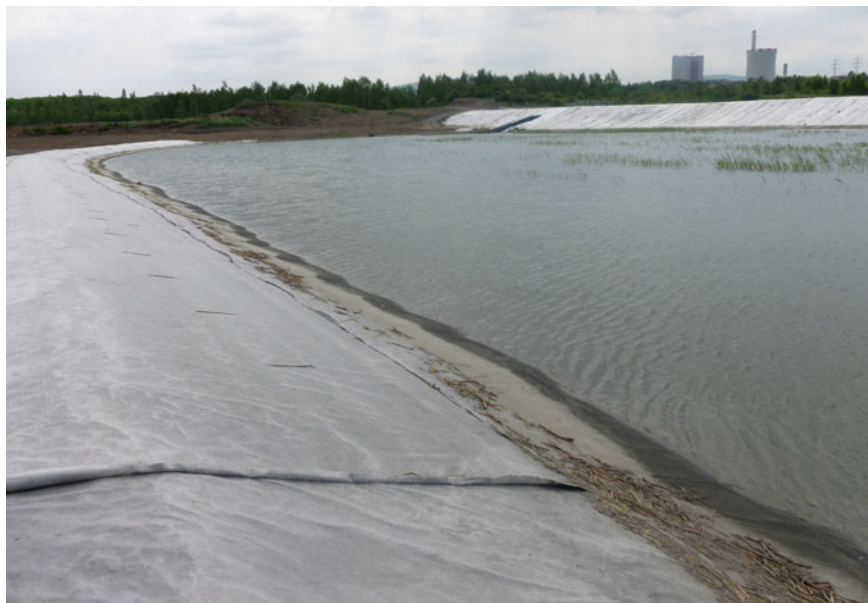
Fig. 7 New earth dike and flooded cassette—a coal power plant in the background
