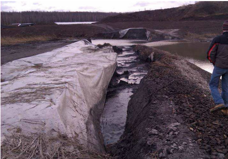
Fig. 3 Damaged earth dike
