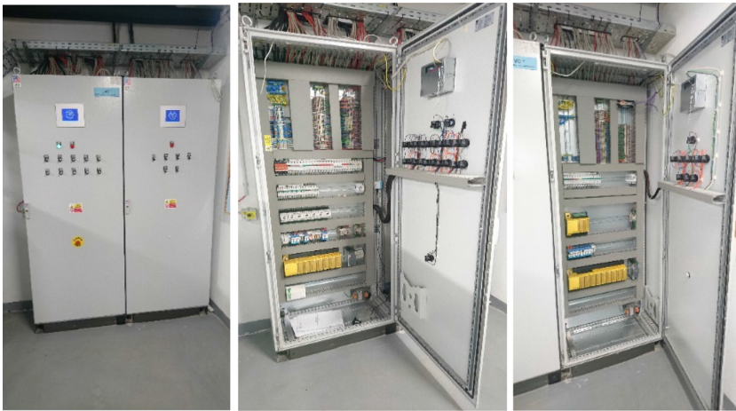
Fig. 5. Base station controlling of heating, cooling and ventilation systems.
