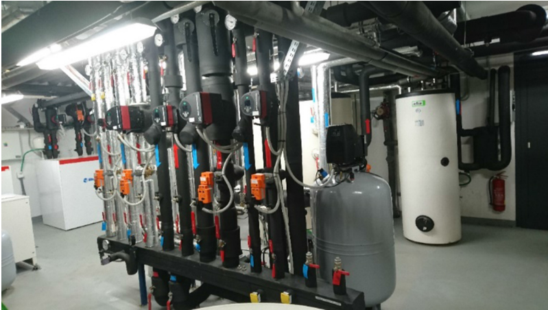
Fig. 3. Distributor and collector of heat and cold to heat exchanger systems of building.
