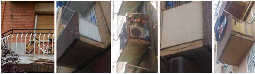
Fig. 26 Damage in balcony slabs
