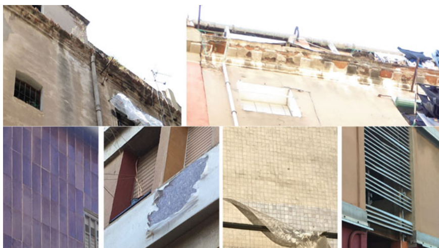
Fig. 29 Material detachment in façades
