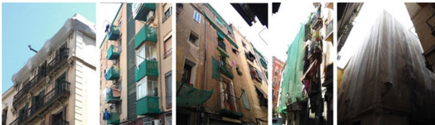
Fig. 14 Buildings with prevention measures applied
