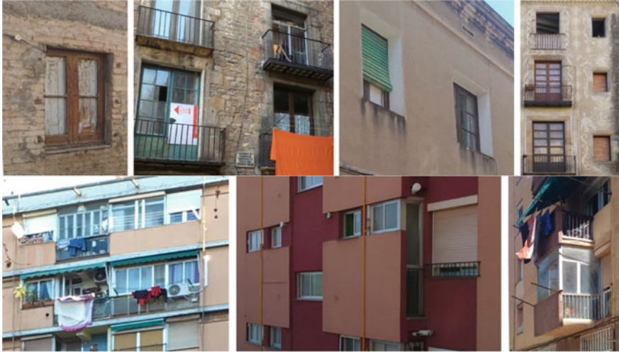
Fig. 33 Damage to carpentry and woodwork in buildings of Type 1 and Type 2 and 4
