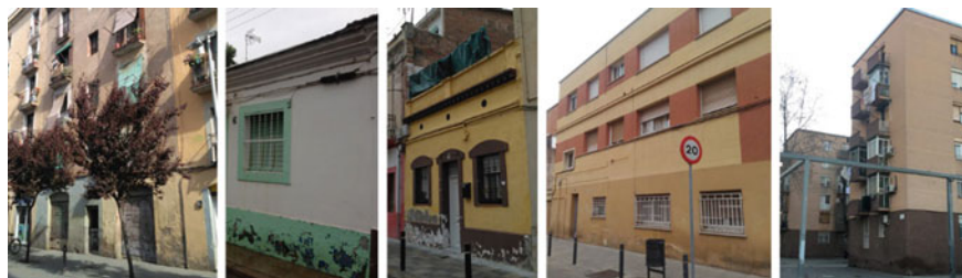
Fig. 16 Cases of rising damp due to capillarity
