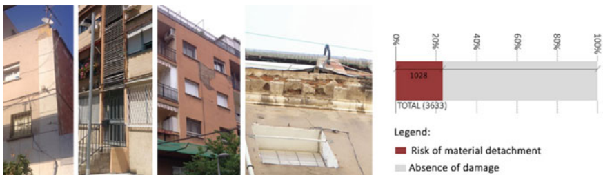
Fig. 13 Presence of unstable façade elements and risk of material detachment and percentage within the total sample
