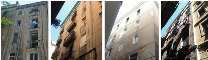
Fig. 27 Cracks and damage in load bearing façades
