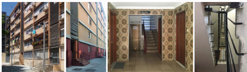
Fig. 36 Accessibility deficiencies in linear blocks of Type 4, in El Besòs neighborhood
