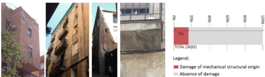
Fig. 12 Presence of damage of mechanical and structural origin and percentage within the total sample
