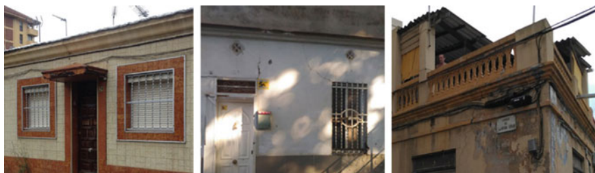
Fig. 24 Cracks in cornices and lintels in type 1 buildings
