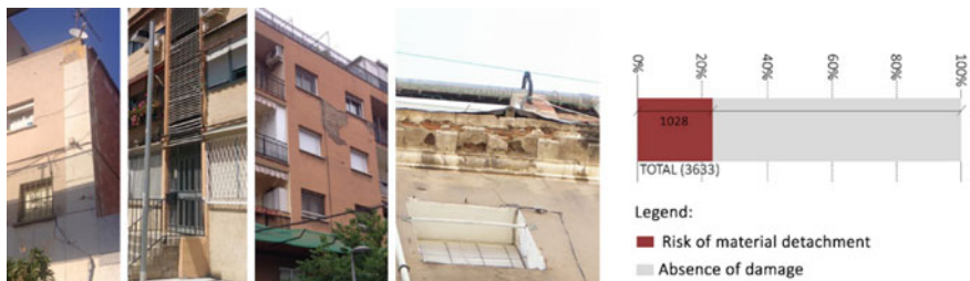
Fig. 13 Presence of unstable façade elements and risk of material detachment and percentage within the total sample
