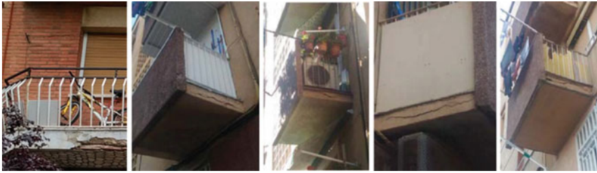
Fig. 26 Damage in balcony slabs
