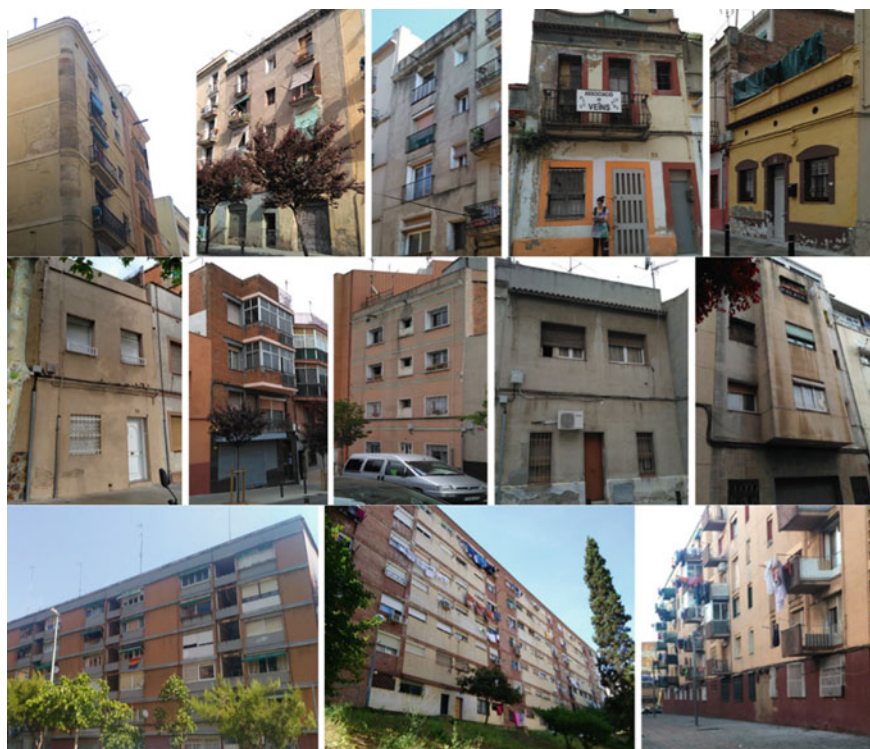
Fig. 31 Damage due to dampness observed in façades. Buildings of Type 1, Type 2 and Type 4
