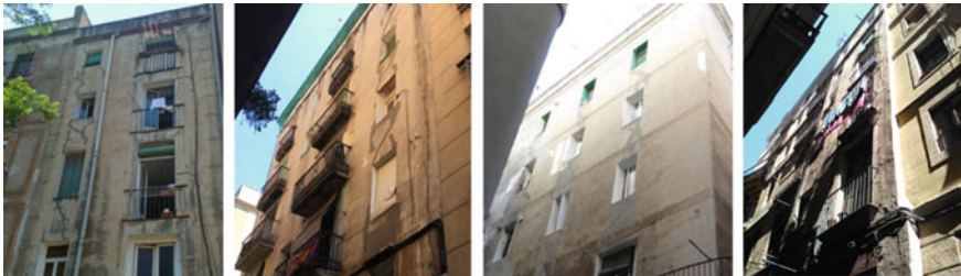
Fig. 27 Cracks and damage in load bearing façades
