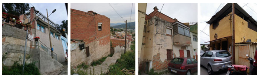
Fig. 25 Damage in type 3 buildings
