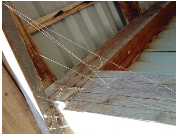
Fig. 5.1 Natural cobweb typically formed under the roofs of the country cottages
