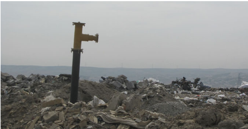
Fig. 2.36 Gas extraction well in place
