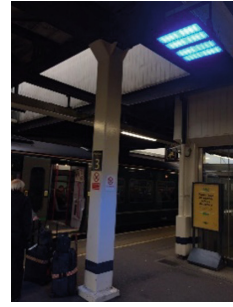
Fig. 7. The blue light illuminating a platform at Horley station near Gatwick Airport, U.K.
