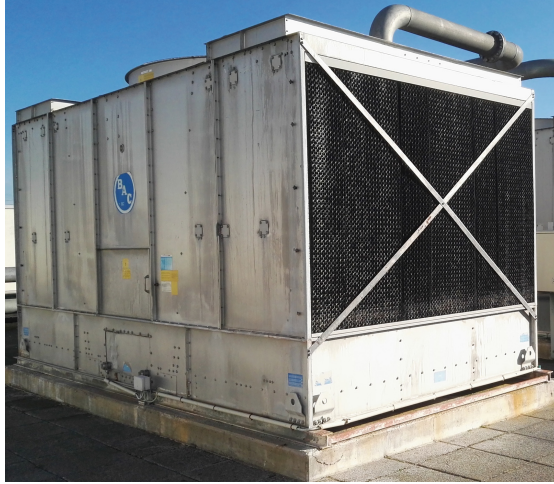
Fig. 3. Photo of cooling tower at the Hospital of León.
