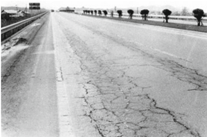
Fig. 5 Severe alligator cracks on the Meishin Expressway
