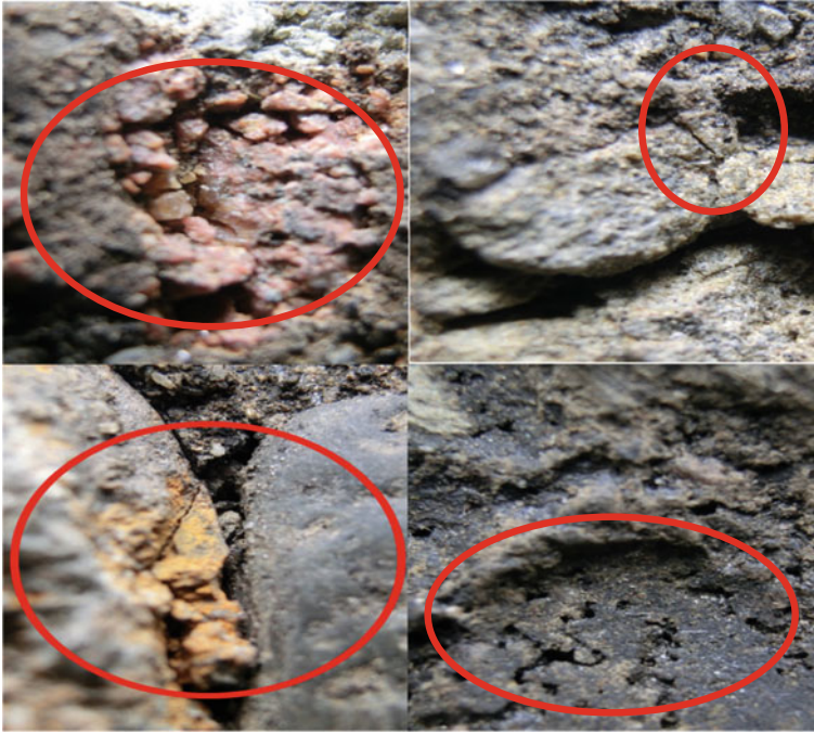
Fig. 8 Examples of crushed, cracked and missing aggregates and mastic in cores from milled pavements
