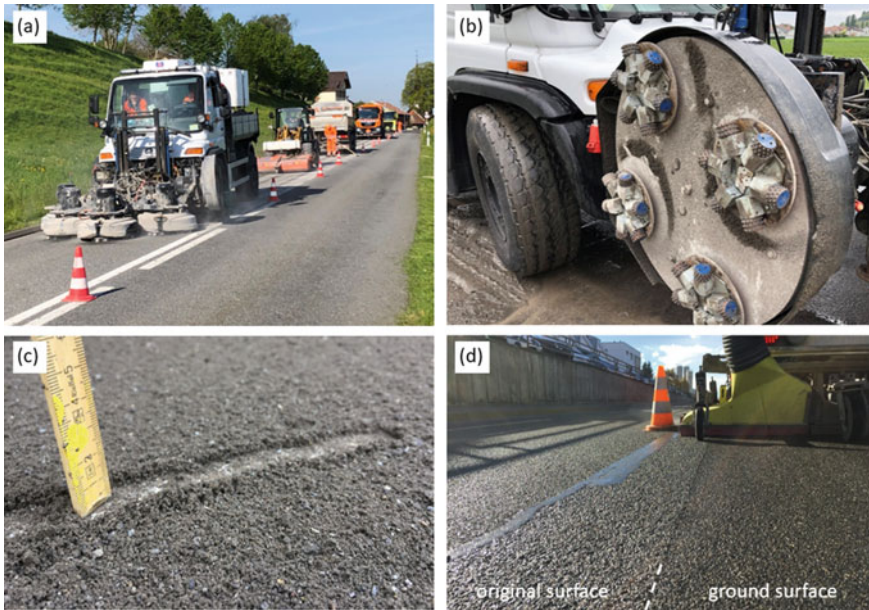
Fig. 1 Images of the large-scale grinding work. The lead vehicle a worked its way on the entire width of one lane. The bush hammer tools on the grinding heads b produced an even layer of fine-graded sand c that was cleaned directly by a series of street cleaners. Behind this convoy, the ground surface was left clean and ready for traffic d
