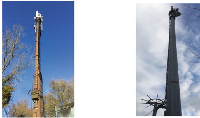
Fig. 3.1 Left. F&Li Monopole. Right. Portasilo monopole
