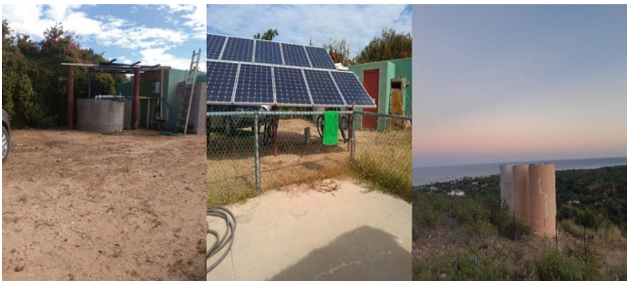
Fig. 28.2 Promotora Pelicano SA de CV's hydraulic infrastructure
