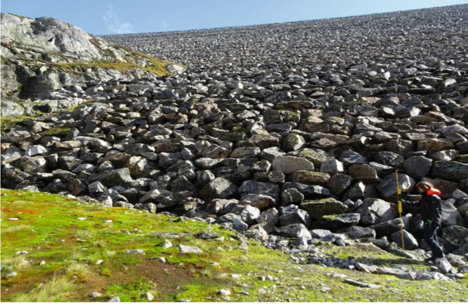
Fig. 1. Depiction of placed riprap constructed on the downstream slope of the 143 m high dam Oddatjørn, highest rockfill dam in Norway. (Photo: NTNU)
