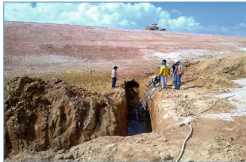
Fig. 6. Piping risk at left abutment of existing dam
