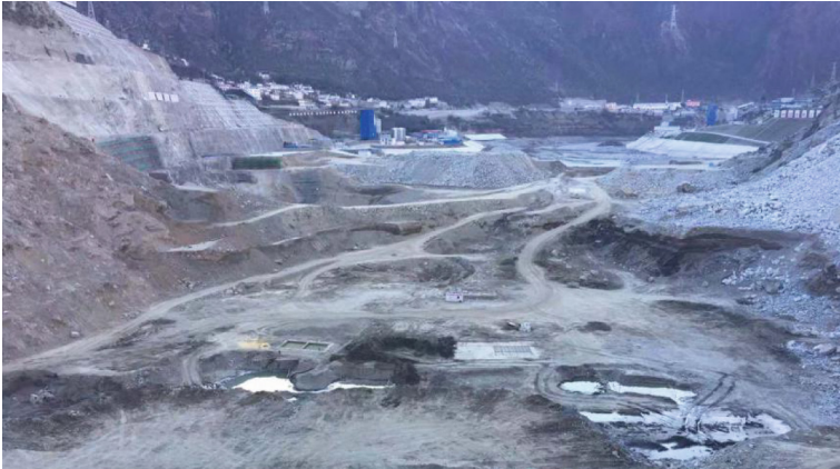
Fig. 3. Destruction and removal of upstream and downstream cofferdams of Suwalong Hydropower Station
