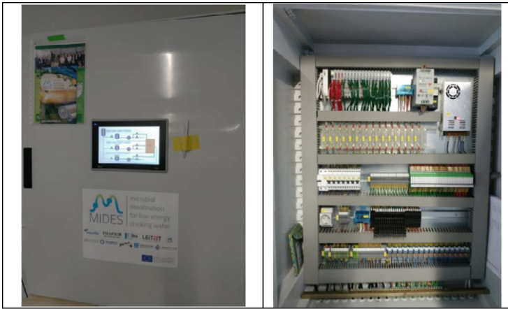
Fig. 11. MIDES pre-pilot control system switchboard: external and internal views.
