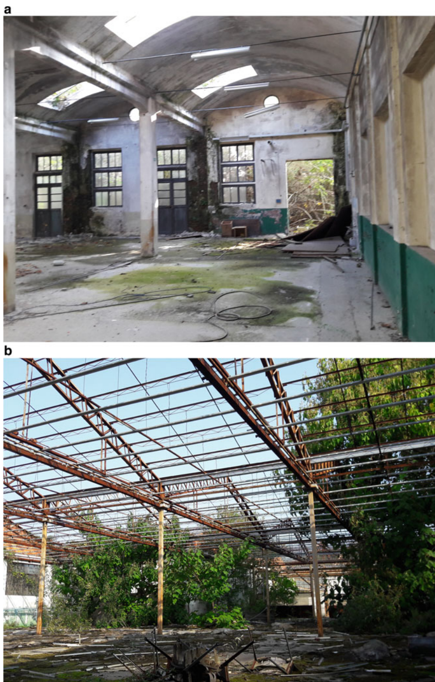
Fig. 7 Former industrial complex in Varese province (Italy). Lowered concrete barrel vaults (a), metal roofing skeleton (b)
