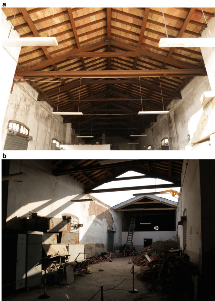
Fig. 1 Former warehouse of the State Railway, Varese (Italy); timber roofing system (a) inner space where the roof is lacking (b). Photographs by Michela Albergati, Federica Borrello, Elena Grisa, Gennaro Merolla, Federico Nunziata, Giulia Turati
