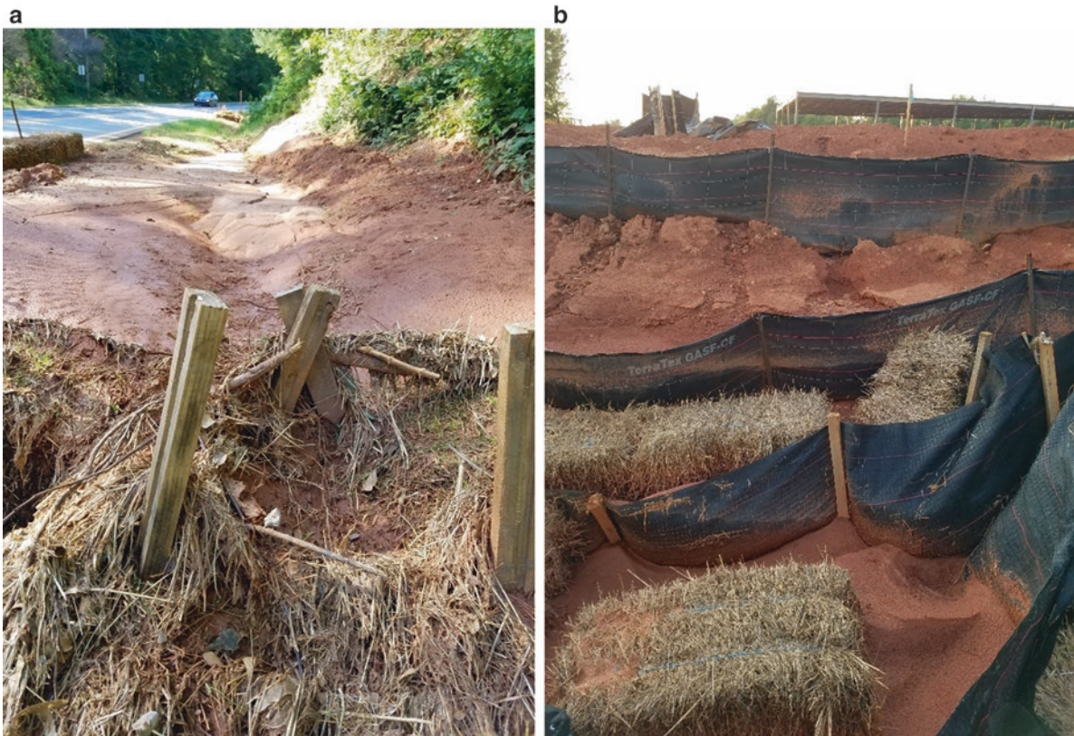
Fig. A5 Examples of erosion of typical Piedmont soils (Ultisols) near Athens, GA, June 2018. (a) Erosion associated with roadside utilities installation, and (b) erosion associated with new commercial construction. In both cases, workers attempted to slow the erosion process. Sediment was nevertheless making its way into local waterways, resulting in overall soil loss (and diminished surface water quality) (Photo credit: Mac Callahan, USDA Forest Service)
