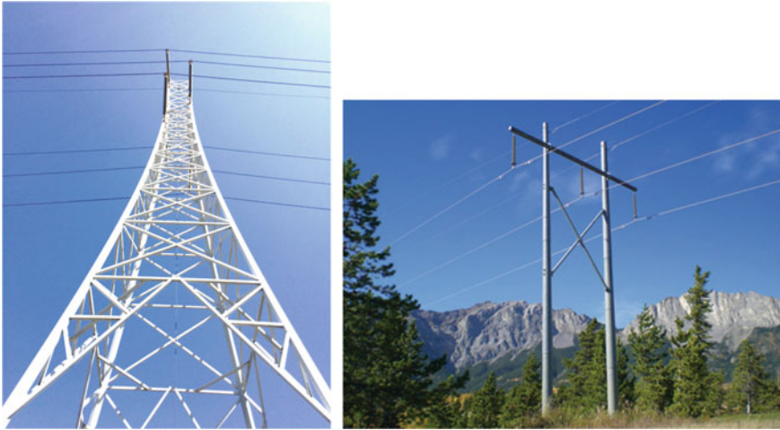
Picture 11 110 kV towers made of composite material. Left: tower in lattice design, right: tower made of tubular poles (Source Cigre Working Group B2.61 “Transmission Line Structures with Fibre Reinforced Polymer (FRP) Composites”)
