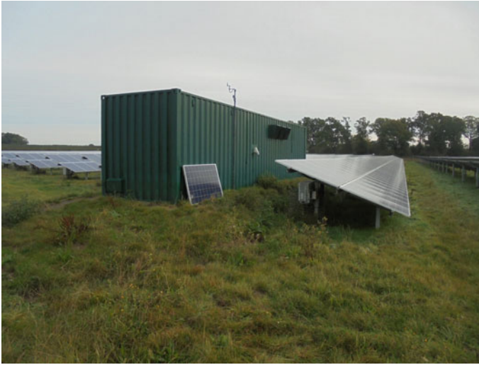
Fig. 4 Container substation, including transformer, for solar integration
