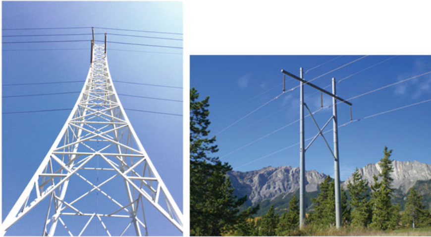
Picture 11 110 kV towers made of composite material. Left: tower in lattice design, right: tower made of tubular poles (Source Cigre Working Group B2.61 “Transmission Line Structures with Fibre Reinforced Polymer (FRP) Composites”)
