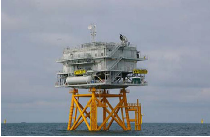
Fig. 5 Walney 1 Offshore substation
