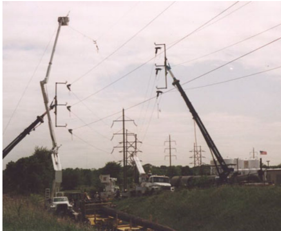
Picture 15 138 kV double dead-end structure replacement utilizing the LineMaster™—Chicago, IL. © Quanta Services [6]
