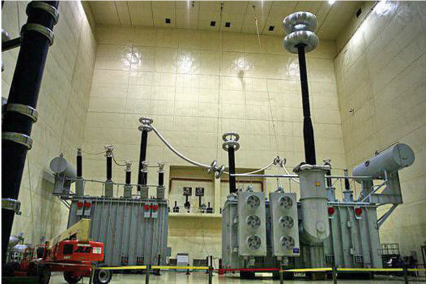
Fig. 6 Typical 1000 kV AC transformer on test
