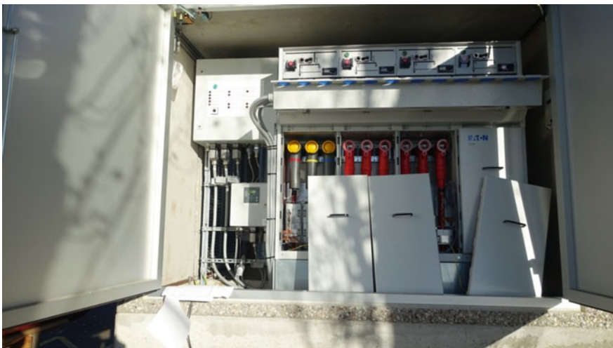
Fig. 13 Tested tele-controlled 12 kV RMU with telecommunication and control box (courtesy of Eaton)
