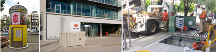
Fig. 18 12 kV RMUs adapted to their environment and automated underground 25 kV switchgear
