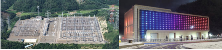
Fig. 3 Ordinary outdoor versus modern indoor substation
