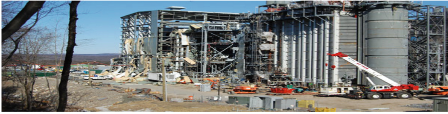
Fig. 1. The Kleen Energy power plant project in Middletown, United States is seen on 7th of February 2010, after explosion [14].
