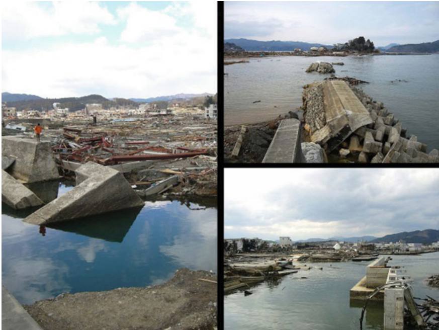
Fig. 12 Seawalls along the coast of the Kesen-numa Port broken by the tsunami on 11 March 2011
