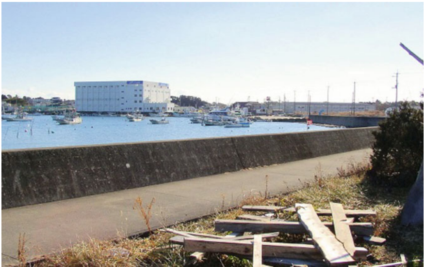
Fig. 9 Picture showing seawall after the Chile Tsunami in 1960
