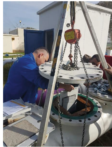
Fig. 4. In-situ exposure of the cement-based lining to the conditions inside the functioning water-supplying pipe line
