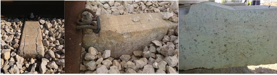
Fig. 1. Characteristic longitudinal cracking on top (left) and side surfaces (center). The net cracking pattern on the surface of a new concrete sleeper (right).
