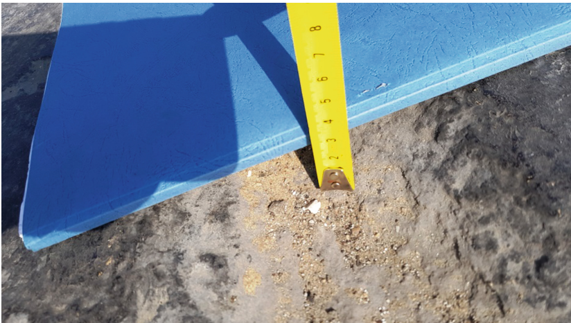
Fig. 3. The depth of maximal pavement's damage after steel scrubs handling
