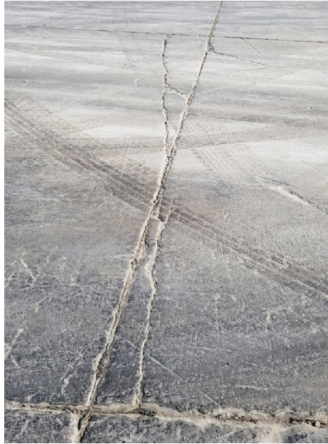
Fig. 6. Cracks next to the saw cut joint
