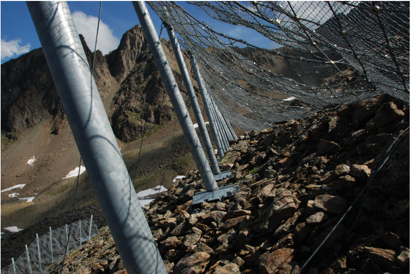
Fig. 28.9 Flexible steel snow nets built on the western flank of Muot da Barba Peider in 2011 with “floating” foundations (steel plates at the ground surface), specially designed for creeping permafrost conditions (photo M. Phillips)
