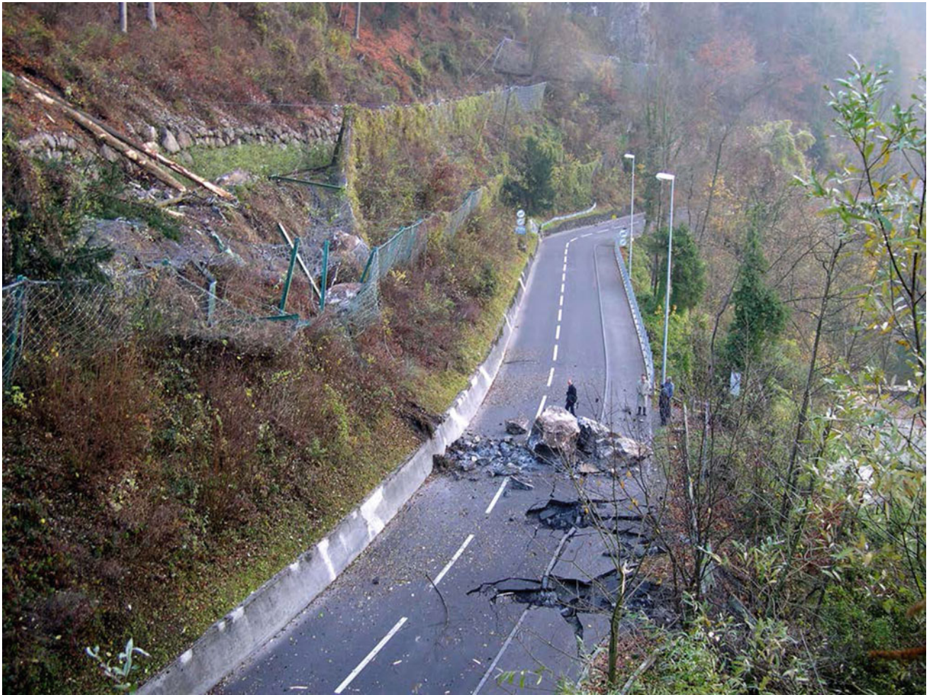
Fig. 21.15 In 2003, a high-energy fragmental rock fall broke through three rows of steel rope nets, causing major damage on the main road south of the town of Vitznau, and some fragments eventually arrested at
