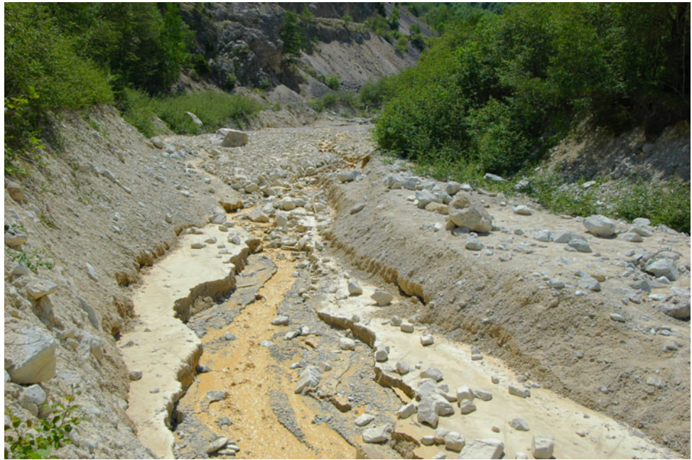
Fig. 25.10 Debris-flow lobe deposit (thickness \sim 2 m) in the channel upstream of the fan apex (photo B. McArdell)
