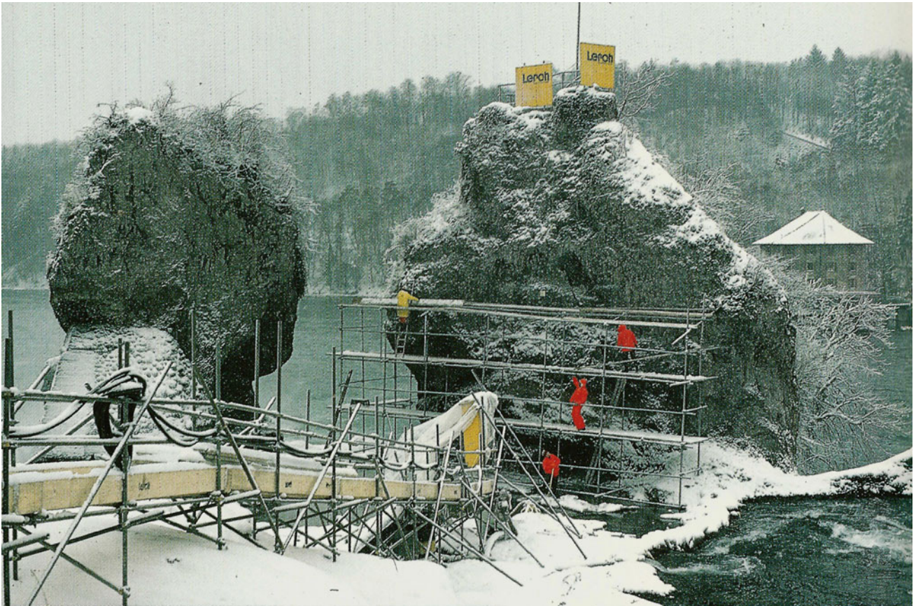
Fig. 23.8 Reinforcement works at the two towers separating the two main falls. The smaller was repaired in winter 1879/80, the bigger during low water in winter 1984/85 (Source Stadtarchiv, J 02.14.01.05/22, Schaffhausen)
