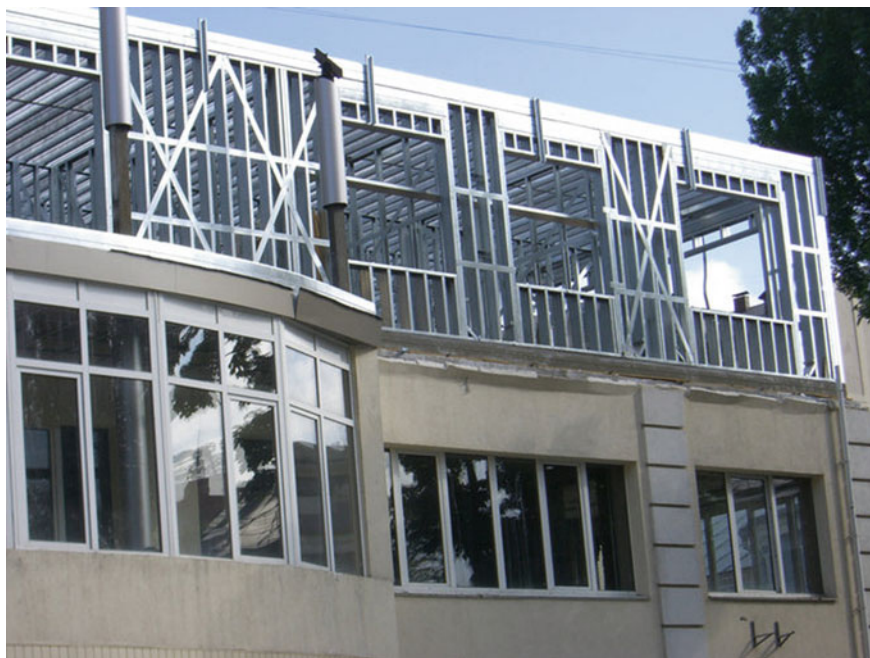
Fig. 8 Reconstruction of the building with an additional storey with lightweight thin-walled metal enclosure structures
