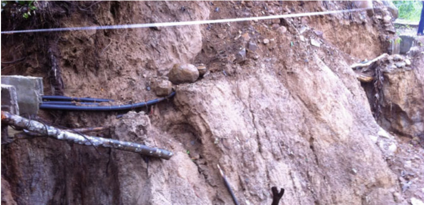
Fig. 16 Damaged portion of the canal due to landslide brought about by heavy rains. Landslide struck the 15-m-long canal located halfway through the total stretch on 2 October 2013, due to heavy downpour. Reconstruction immediately started on 10 October 2013
