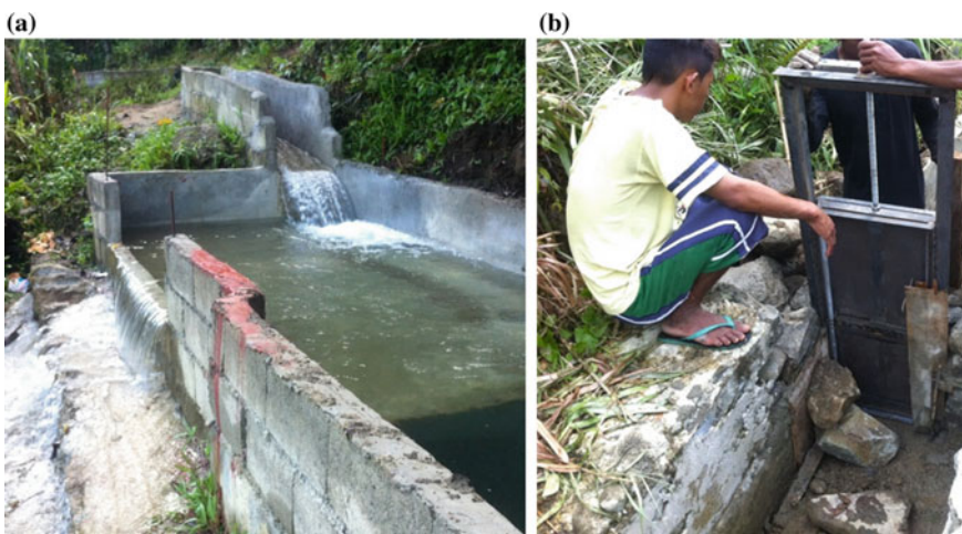
Fig. 18 a Forebay spillway and b intake flood control gate
