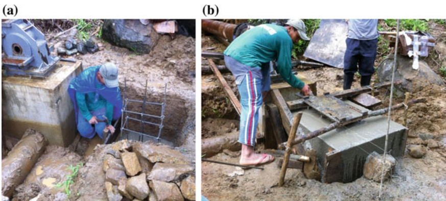
Fig. 23 a Setting the generator foundation using reinforced steel bars and b curing of concrete
