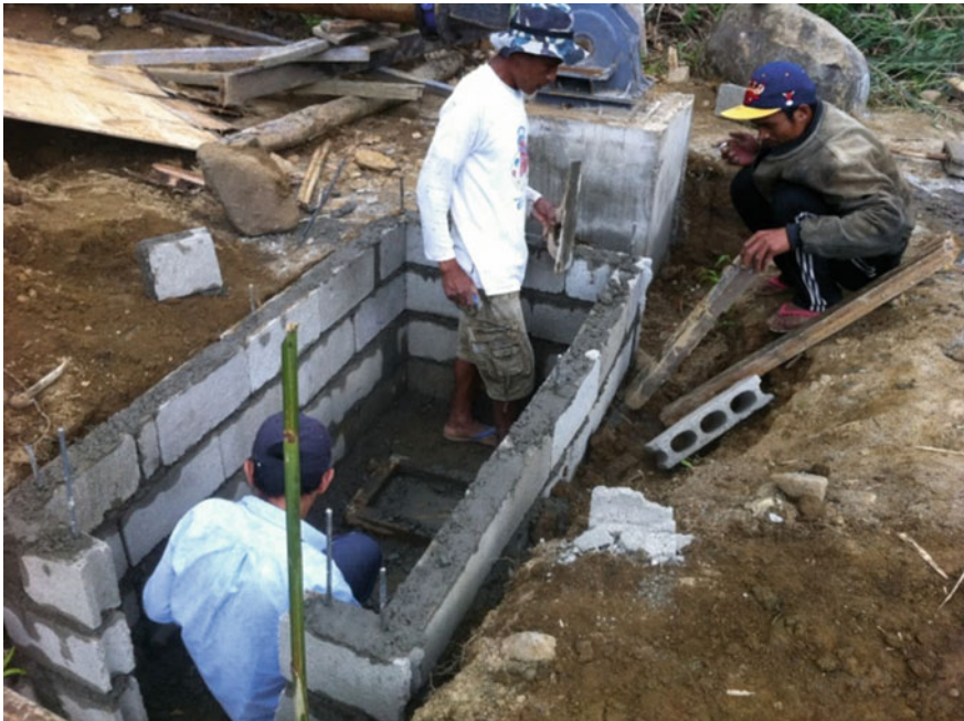
Fig. 25 Tailrace canal with open rectangular weir for flow measurement
