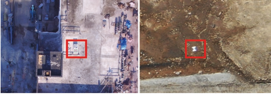
Fig. 5.4 Example of GCPs (marked in red) place on the construction site for registering the Reality models to BIM or real-world coordinate system
