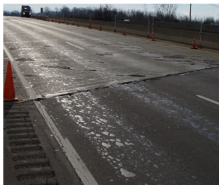
(a) Deck Spalling on North Abutment
