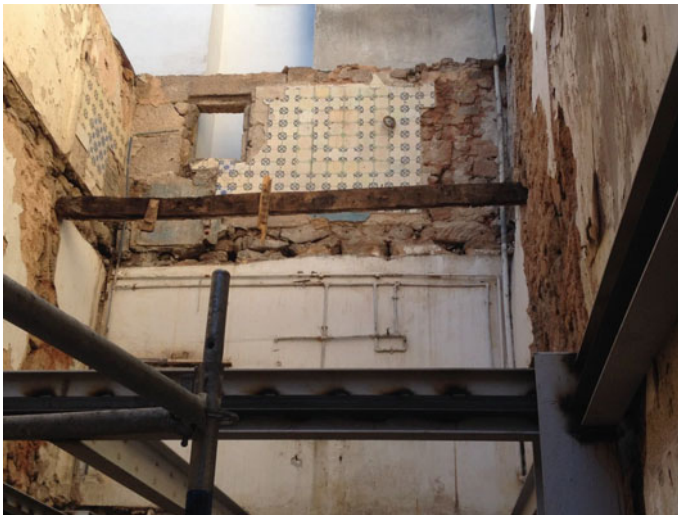
Fig. 1 General appearance of the interior of the building after demolition of its interior
